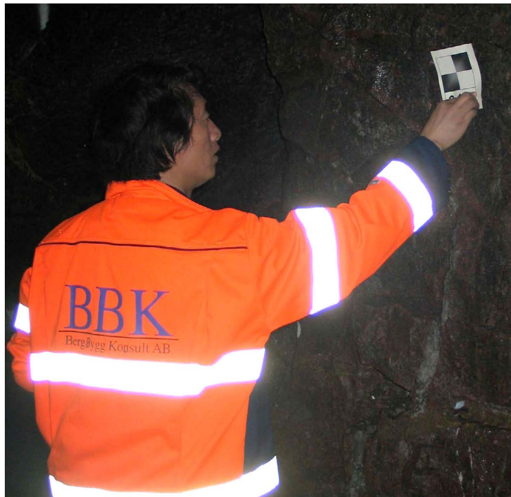
Reference markers are put up on the tunnel wall before the laser scanning can begin.
