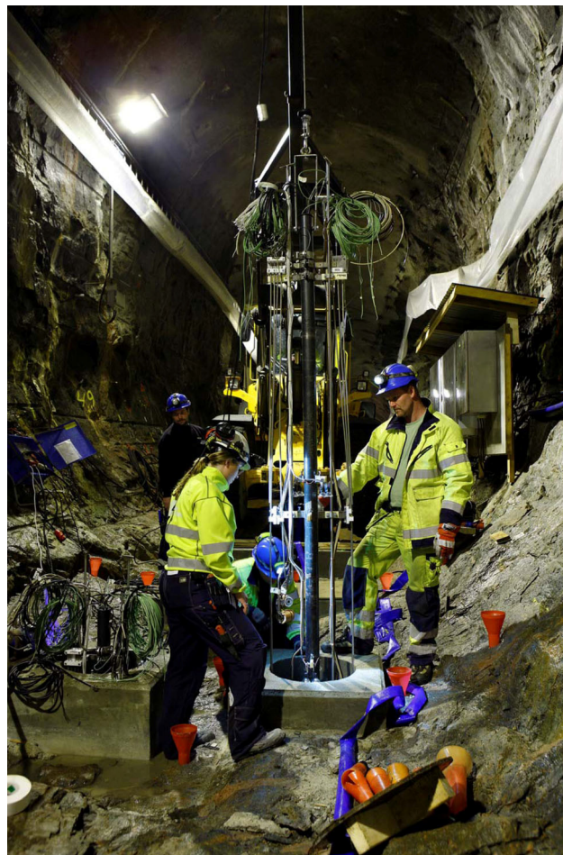
Figure 2-1. Installation of test equipment in the first test within the Caps field experiment in the Tasq-tunnel.
